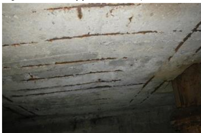
Figura 4.23. Plafonul cuvei umede – cu armatura la vedere (2017) Figure 4.23. The ceiling of the wet tub – with the reinforcement visible (2017)
