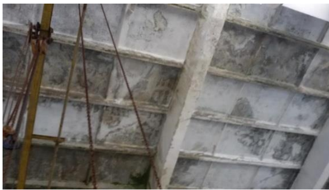
Figura 4.16. Planșeu Stație de pompare – degradat (2017) Figure 4.16. Floor Pumping station – degraded (2017)
